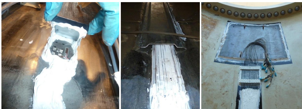
Figure 6: adhesive-based pile instrumentation with encapsulation for sensors (left), steel profile covering sensors and cables (middle) and mounting plate for DAQ unit (right)
