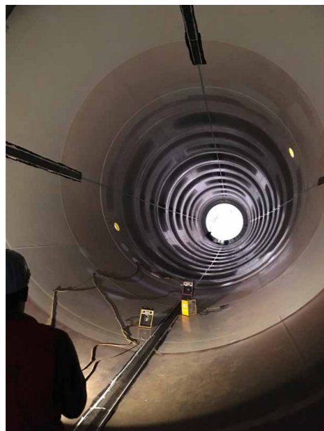
This Side: Instrumentation inside a Monopile (Photo IGB) Rock Salt after load test (Photo IGB)
